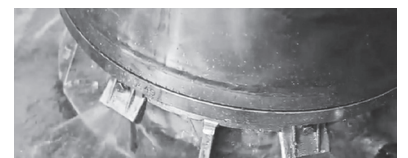
Hydraulic barrier to keep fibre out
